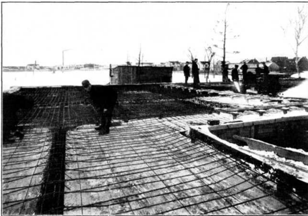
PLATE IV, FIG. 2.—REINFORCEMENT IN PLACE OVER ONE COMPLETE FLOOR OF STORAGE WAREHOUSE. SLABS, 14 FT. SQUARE. REINFORCED TWO WAYS. NOTE CONTINUITY OF REINFORCEMENT AND ELEVATION OVER SUPPORTS. FLOOR DESIGNED FOR 150 LB. PER SQ. FT. LIVE LOAD. TESTED TO 900 LB. PER SQ. FT.
