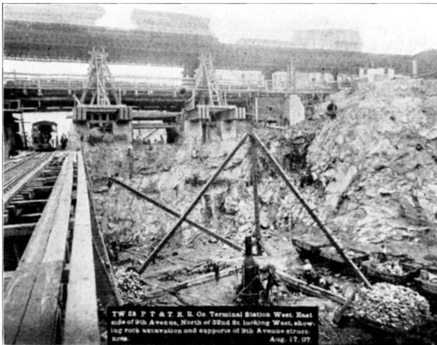
PLATE XLVII, FIG. 4.— TW 28, P.T. & T.R.R. CO. TERMINAL STATION WEST. EAST SIDE OF 9TH AVENUE, NORTH OF 32ND ST. LOOKING WEST, SHOWING ROCK EXCAVATION AND SUPPORTS OF 9TH AVENUE STRUCTURES. AUG. 17, 07.
