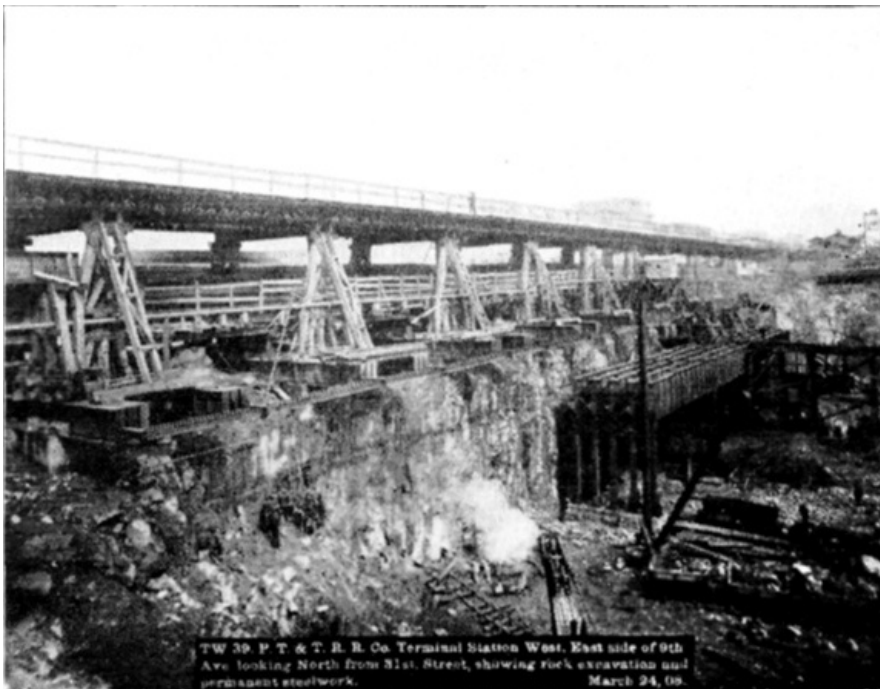
PLATE XLVIII, FIG. 2.— TW 39, P.T. & T.R.R. CO. TERMINAL STATION WEST. EAST SIDE OF 9TH AVE. LOOKING NORTH FROM 31ST STREET, SHOWING ROCK EXCAVATION AND PERMANENT STEEL WORK. MARCH 24, 08.
