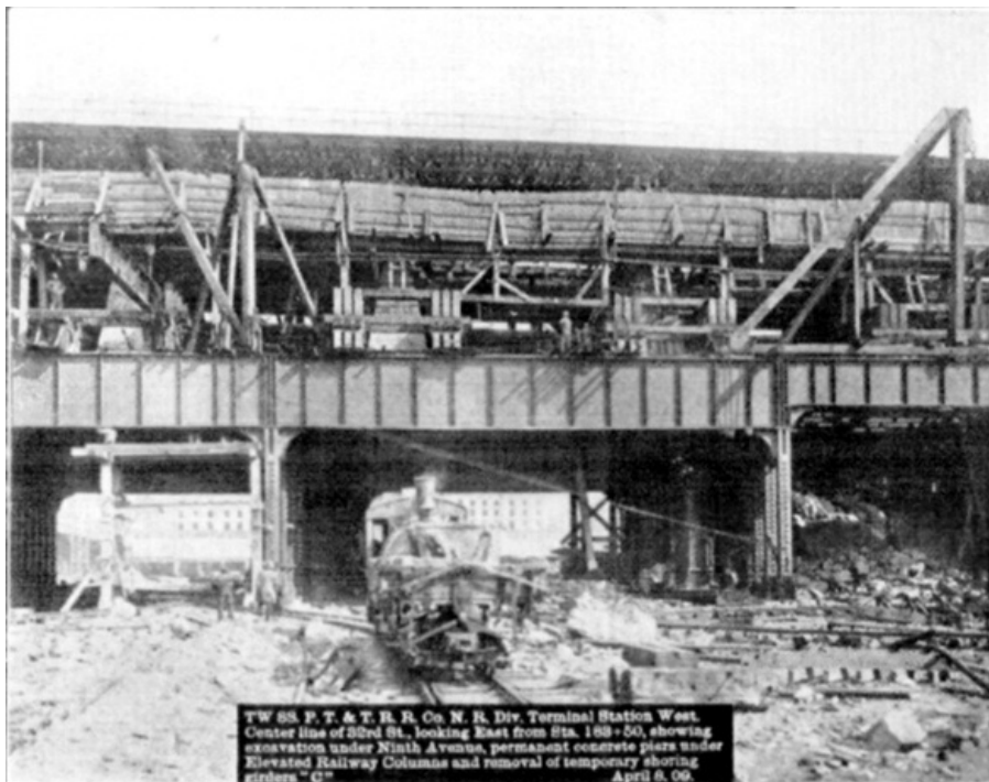
PLATE XLIX, FIG. 3.— TW 88, P.T. & T.R.R. Co. N.R. Div. TERMINAL STATION WEST. CENTER LINE OF 32ND ST., LOOKING EAST FROM STA. 183+50, SHOWING EXCAVATION UNDER NINTH AVENUE, PERMANENT CONCRETE PIERS UNDER ELEVATED RAILWAY COLUMNS AND REMOVAL OF TEMPORARY SHORING GIRDERS "C". APRIL 8, 09.
