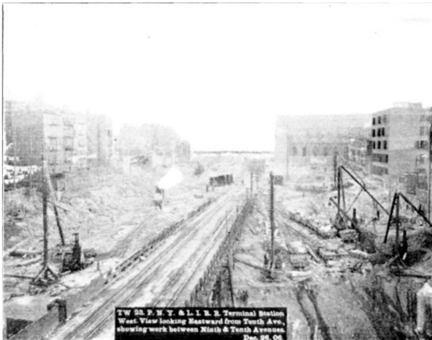
PLATE L, FIG. 1.— TW 23, P.N.Y. & L.I.R.R. TERMINAL STATION WEST. VIEW LOOKING EASTWARD FROM TENTH AVE., SHOWING WORK BETWEEN NINTH & TENTH AVENUES. DEC. 26, 06.
