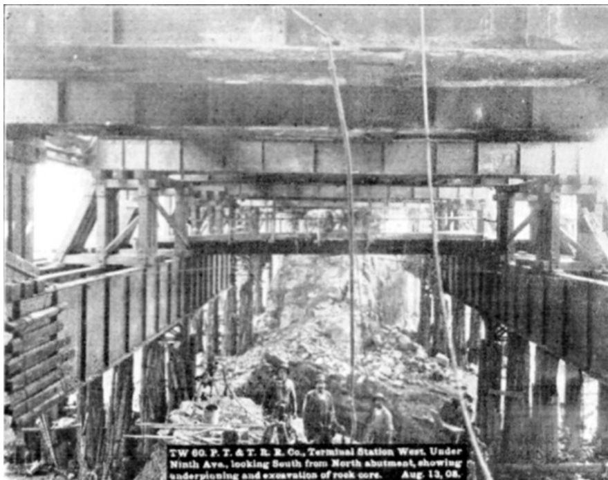
PLATE XLIX, FIG. 1.— TW 60, P.T. & T.R.R. Co. TERMINAL STATION WEST. UNDER NINTH AVE., LOOKING SOUTH FROM NORTH ABUTMENT, SHOWING UNDERPINNING AND EXCAVATION OF ROCK CORE. AUG. 13, 08.
