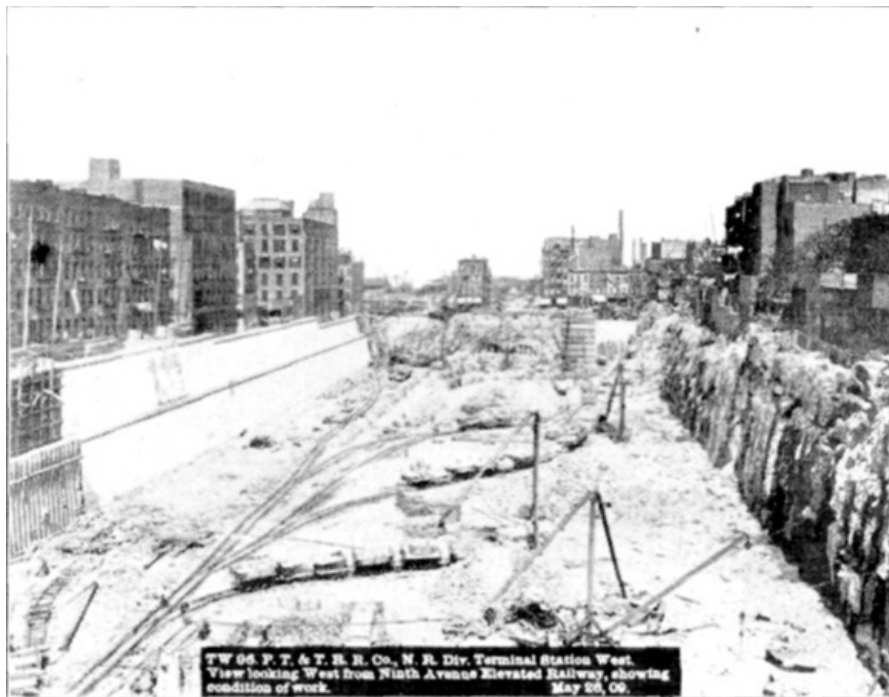
PLATE L, FIG. 3.— TW 96, P.T. & T.R.R. CO. N.R. DIV. TERMINAL STATION WEST. VIEW LOOKING WEST FROM NINTH AVENUE ELEVATED RAILWAY, SHOWING CONDITION OF WORK. MAY 26, 09.
