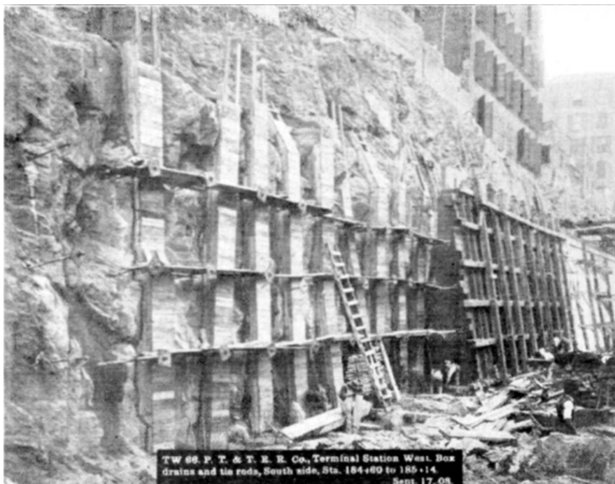
PLATE LI, FIG. 1.— TW 66, P.N.Y. & L.I.R.R. TERMINAL STATION WEST. BOX DRAINS AND TIE RODS, SOUTH SIDE, STA. 184+80 TO 185+14. SEPT. 17, 08.
