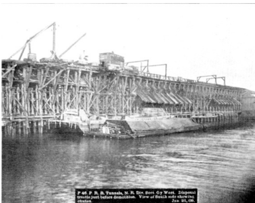
PLATE LI, FIG. 3.— P 46. P.R.R. TUNNELS, N.R. DIV. SECT. GY. WEST. DISPOSAL TRESTLE JUST BEFORE DEMOLITION. VIEW OF SOUTH SIDE SHOWING CHUTES. JAN. 21, 09.
