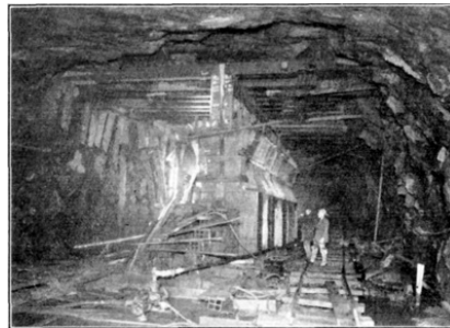
PLATE LX, FIG. 2.—CENTER WALL AND SKEWBACK UNDER I-BEAMS, AFTER REMOVAL OF DOUBLE ROW OF POSTS.
