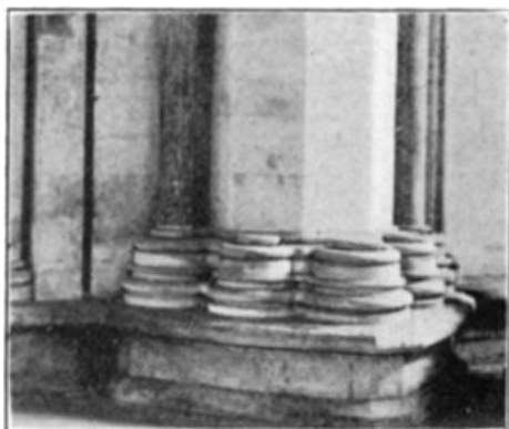
BASE OF INCOMPLETE PIER.
