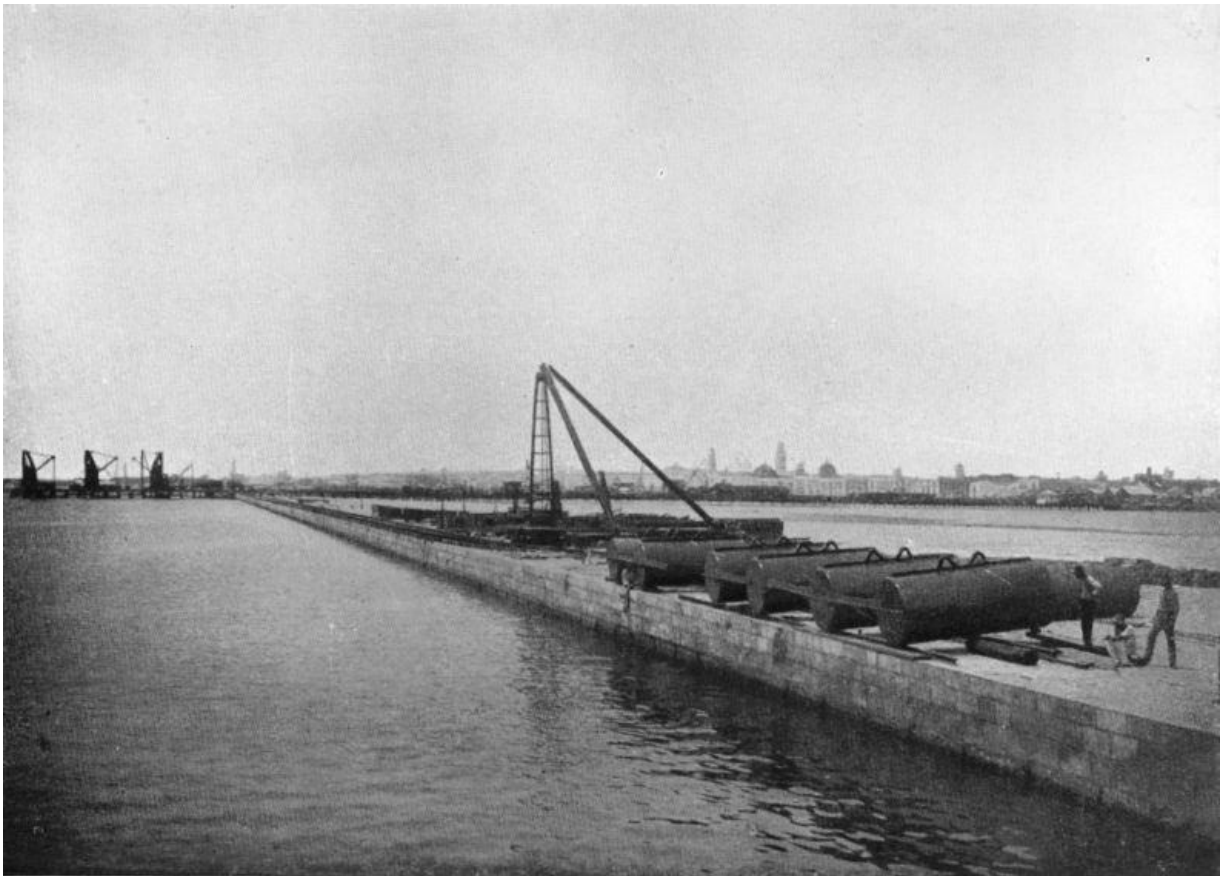
MEXICO'S ARTIFICIAL HARBOURS: THE NEW PORT WORKS AT VERA CRUZ, A SOLID AND COSTLY ENTERPRISE.
