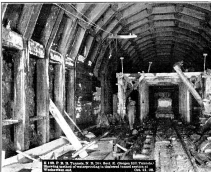
FIG. 4. K 168. P.R.R. Tunnels, N. R. Div. Sect. K. (Bergen Hill Tunnels.) Showing method of waterproofing in timbered tunnel section at Weehawken end. Oct. 21, 08.
