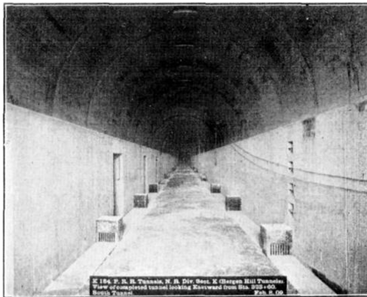
FIG. 2. K 184. P.R.R. Tunnels, N. R. Div. Sect. K. (Bergen Hill Tunnels). View of completed tunnel looking Eastward from Sta. 323+60. South Tunnel. Feb. 8, 09.
