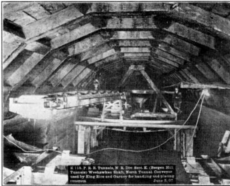
FIG. 3. K 115. P.R.R. Tunnels, N. R. Div. Sect. K. (Bergen Hill Tunnels) Weehawken Shaft, North Tunnel Conveyor used by King Rice and Garney for handling and placing concrete. June 3, 07.
