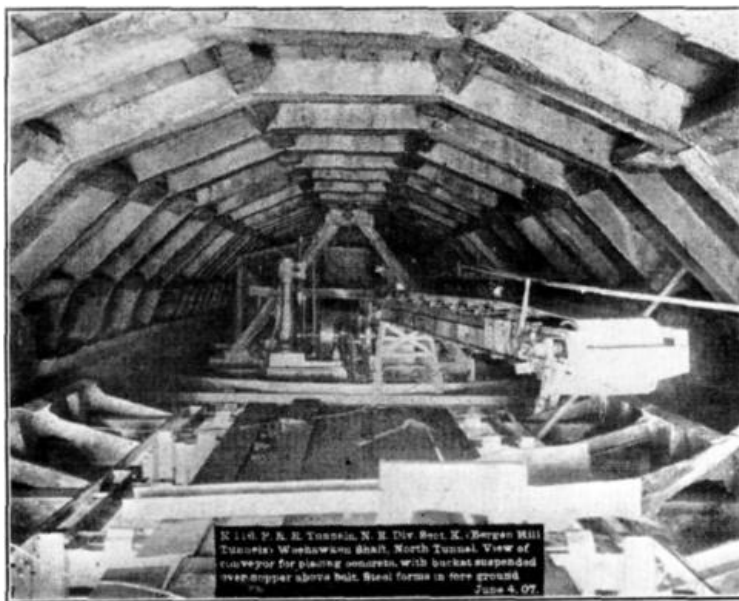
FIG. 4. K 116. P.R.R. Tunnels, N. R. Div. Sect. K. (Bergen Hill Tunnels) Weehawken Shaft, North Tunnel. View of conveyor for placing concrete, with bucket suspended over hopper above belt. Steel forms in fore ground. June 4, 07.
