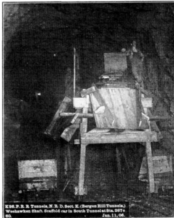
FIG. 1. K 26. P.R.R. Tunnels, N. R. D. Sect. K. (Bergen Hill Tunnels,) Weehawken Shaft. Scaffold car in South Tunnel at Sta. 267+60. Jan. 11, 06.
