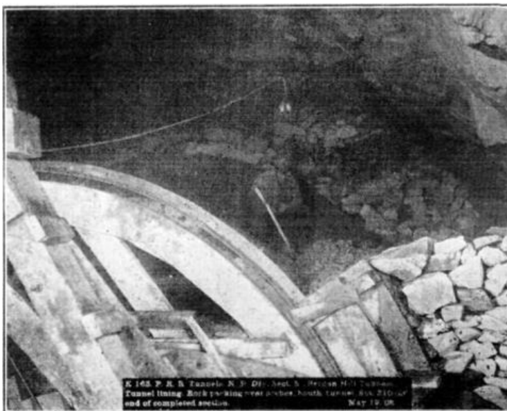
FIG. 3. K 163. P.R.R. Tunnels, N. R. Div. Sect. K. (Bergen Hill Tunnels.) Tunnel lining. Rock packing over arches, South tunnel Sta. 210+00 end of completed section. May 19, 08.
