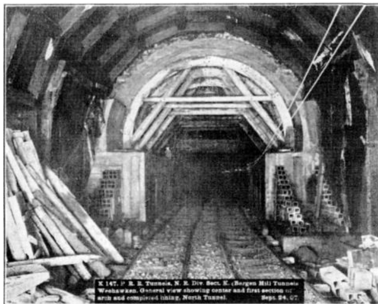
FIG. 4. K 147. P.R.R. Tunnels, N. R. Div. Sect. K. (Bergen Hill Tunnels) Weehawken. General view showing center and first section of arch and completed lining, North Tunnel. Sept. 24, 07.
