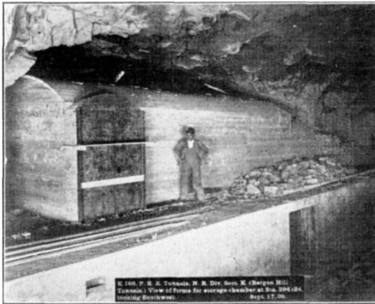
FIG. 2. K 166. P.R.R. Tunnels, N. R. Div. Sect. K. (Bergen Hill Tunnels.) View of forms for storage chamber at Sta. 294+24, looking Southward. Sept. 17, 08.
