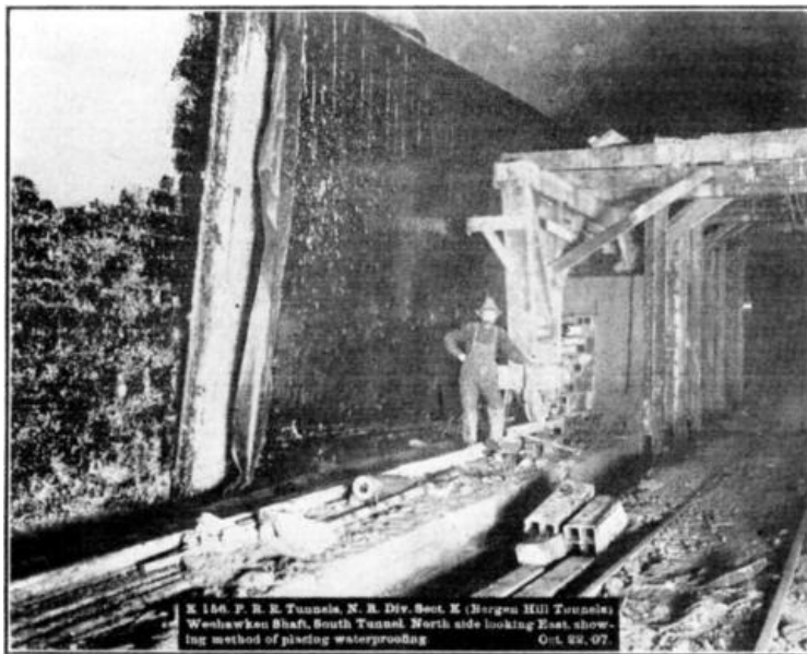
FIG. 3. K 156. P.R.R. Tunnels, N. R. Div. Sect. K. (Bergen Hill Tunnels) Weehawken Shaft, South Tunnel. North side looking East, showing method of placing waterproofing. Oct. 22, 07.
