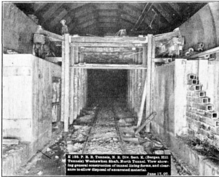
FIG. 2. K 125. P.R.R. Tunnels, N. R. Div. Sect. K. (Bergen Hill Tunnels) Weehawken Shaft, North Tunnel. View showing general construction of tunnel lining forms, and clearance to allow disposal of excavated material. June 17, 07.
