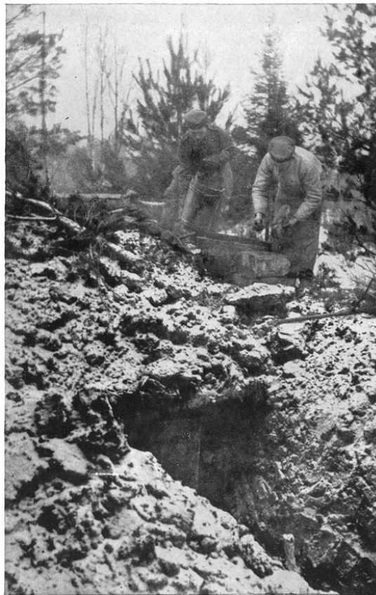
These soldiers have completed their underground shelter by constructing a fireplace and are now adding the finishing touches to the chimney
