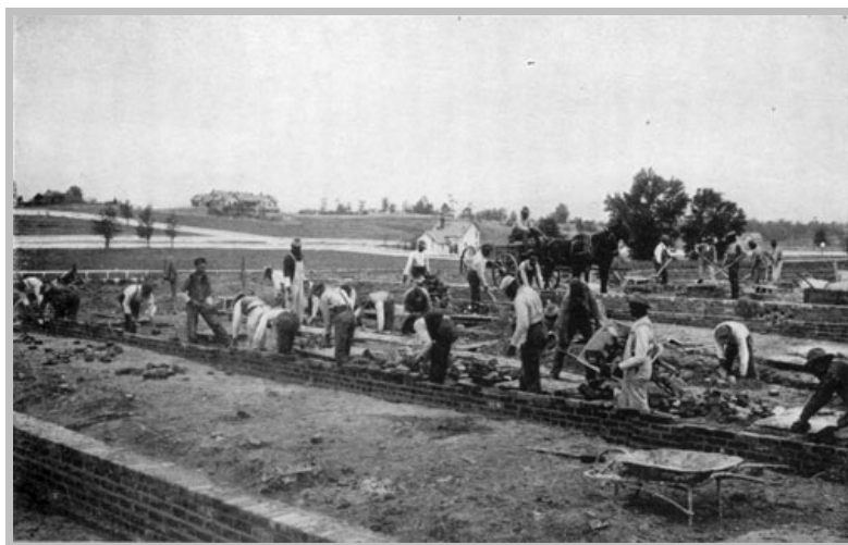
Tuskegee Institute students laying the foundation for one of the four Emery buildings—boys' dormitories.
