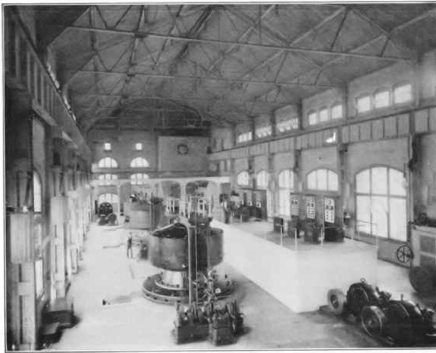
NIAGARA POWER-HOUSE (INTERIOR)
