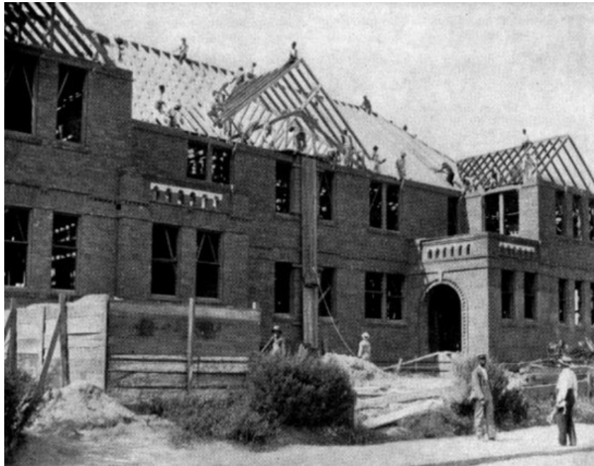
THE OFFICE BUILDING IN PROCESS OF ERECTION. Student carpenters shown at work.
