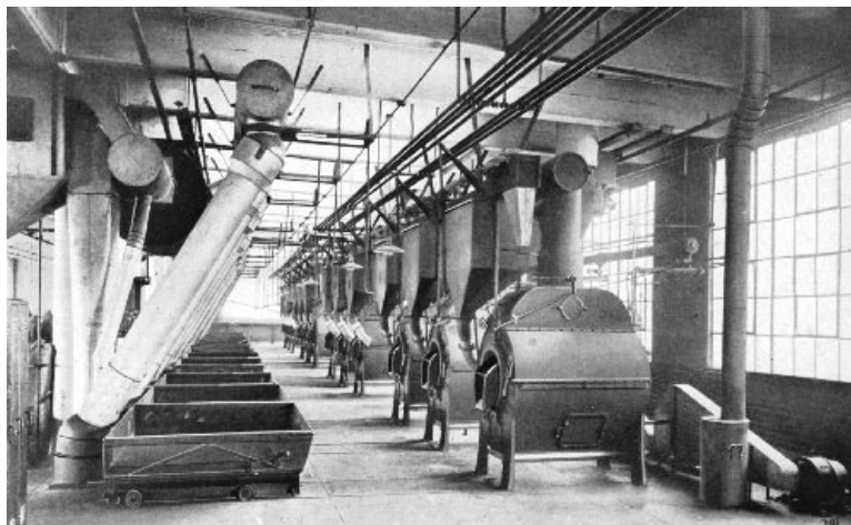
A MODERN GAS COFFEE-ROASTING PLANT WITH A CAPACITY OF 1,000 BAGS A DAY
