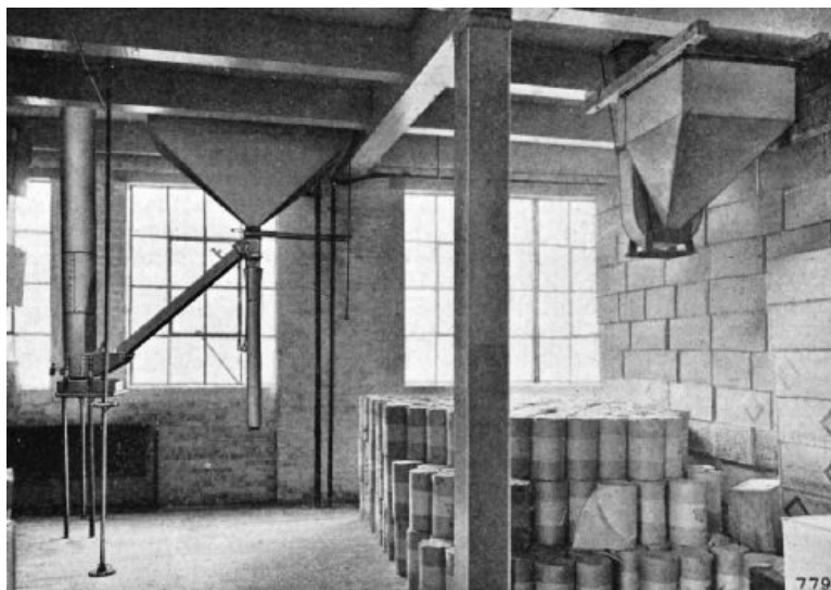
LOWER-STORY VIEW OF THE SAME PLANT FROM ABOUT THE SAME ANGLE Showing connection from floor hopper to stoner on the left, and suspended bucket-elevator boot with four-bag dump hopper on the right COMPLETE GAS COFFEE-PLANT INSTALLATION
