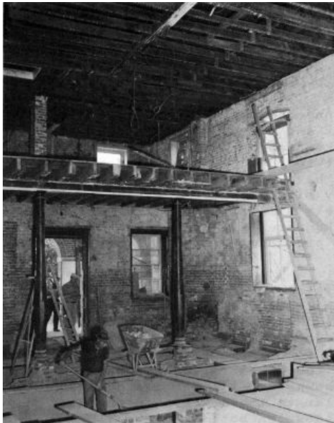
Interior of the gutted courthouse during restoration in 1966. Photo by Lee Hubbard.
