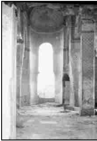
THE MYRELAION (SINCE IT WAS BURNT). INTERIOR, LOOKING EAST. (By kind permission of H. M. Dwight, Esq.)
