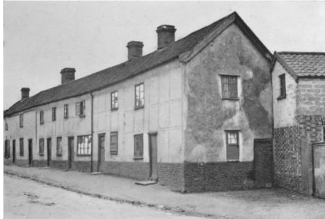
A ROW OF CLAY-LUMP COTTAGES. The front has been plastered and panelled out. In the upper part of the stable building, seen in the foreground, the clay-lumps are shown exposed.
