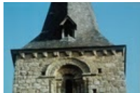
188. Saint-Loup. The Romanesque tower. The cornice rests on modillions carved with human heads or molded in quarter-round. Most of the cornice was rebuilt during the rebuilding of the octagon spire on a square base, with skylights. Photo by Alain Dermigny. [Alain-103]
