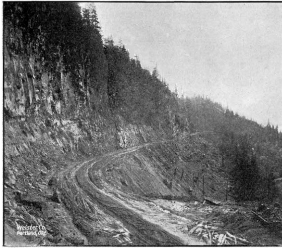
HEAVY GRADING ON RUTHTON HILL IN HOOD RIVER COUNTY. CONSTRUCTED IN 1917 AND 1918
