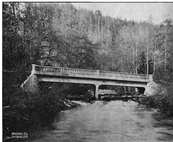
ONE OF NINE REINFORCED CONCRETE BRIDGES IN THE BEAVER CREEK VALLEY, COLUMBIA COUNTY, ON THE COLUMBIA RIVER HIGHWAY BETWEEN RAINIER AND CLATSKANIE. ALL BUILT IN 1917 AND 1918
