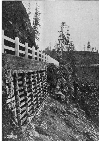
REINFORCED CONCRETE CRIBBING NEAR PRESCOTT ON THE COLUMBIA RIVER HIGHWAY IN COLUMBIA COUNTY. BUILT IN 1918
