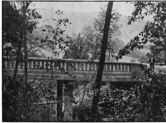
VAN TYNE CREEK VIADUCT NORTH OF MYRTLE CREEK IN DOUGLAS COUNTY. BUILT IN 1918
