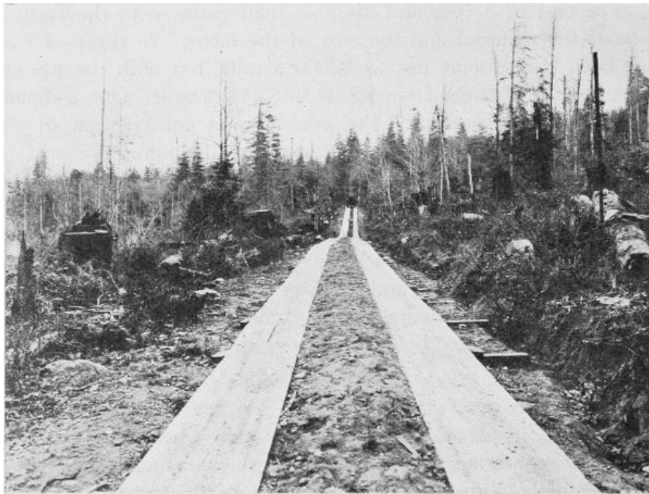
Fore-and-aft plank road with wedges on cross ties to facilitate the re-aligning of the planks.
