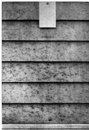
Hail-stone Abrasions on House Repainting Tests
