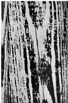
SCALING.—Type of Decay Exhibited by Improperly Made Paint (magnified view)
