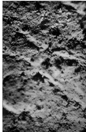
CHALKING.—Type of Decay Exhibited by Improperly Made Paint (magnified view)
