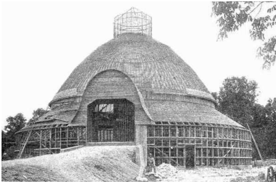
FIG. 39. SHOWING CONSTRUCTION OF BARN IN FIG. 40. HOOPS IN PLACE READY FOR PERPENDICULAR SIDING; ROOF SHEATHED FOR SHINGLES.
