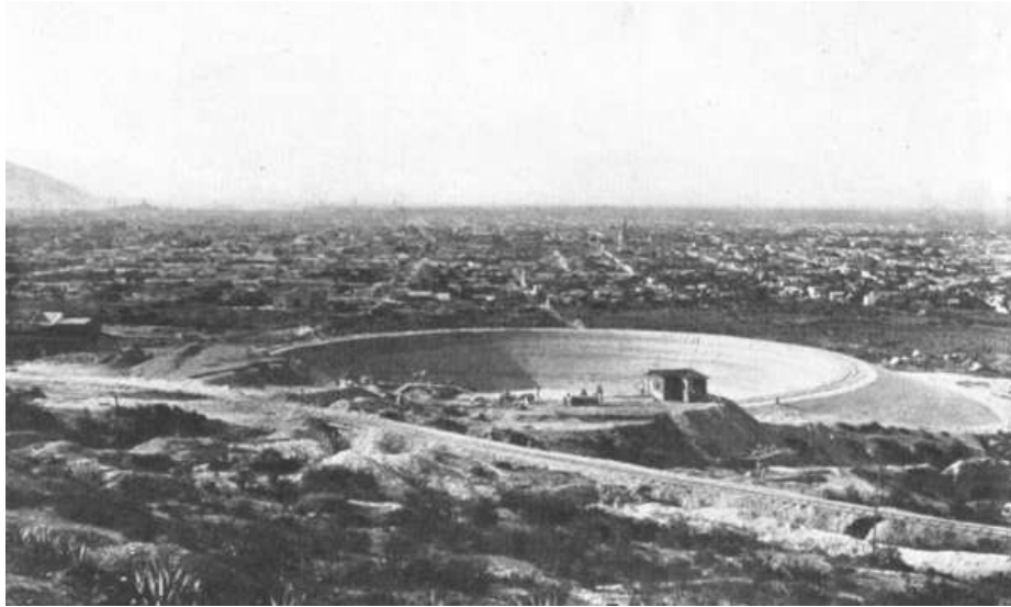
PLATE VIII, FIG. 1.—GENERAL VIEW OF EXCAVATION AND EMBANKMENT FOR SOUTH RESERVOIR BEFORE LINING.
