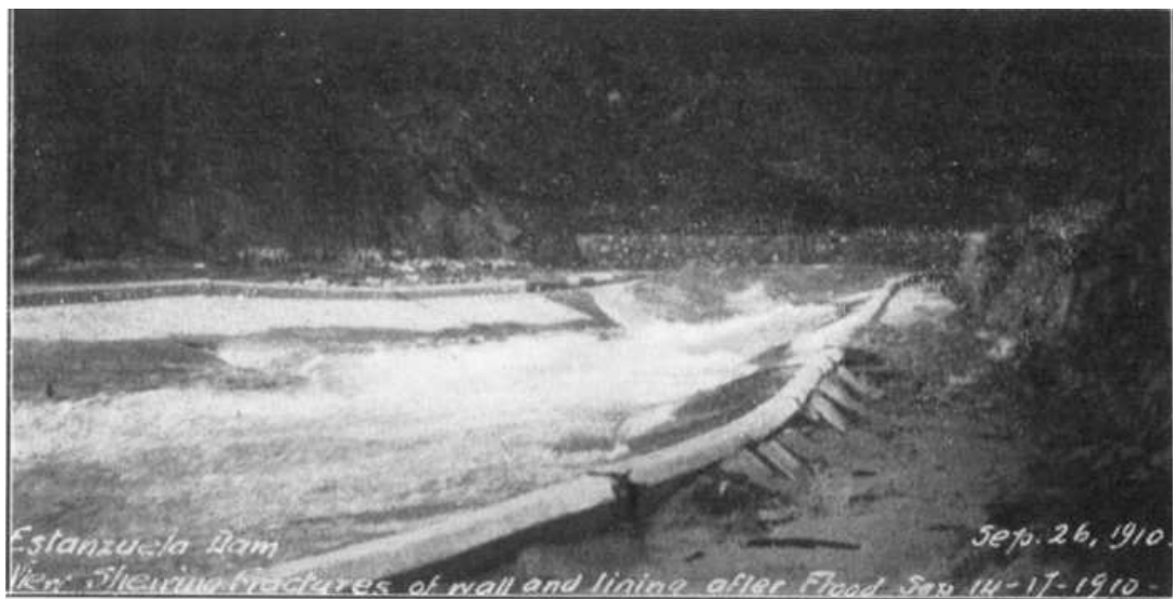
PLATE XXXIII, FIG. 3.—ESTANZUELA DAM SEPT. 26, 1910: VIEW OF SHEARING FRACTURES OF WALL AND LINING AFTER FLOOD SEPT. 14-17, 1910.
