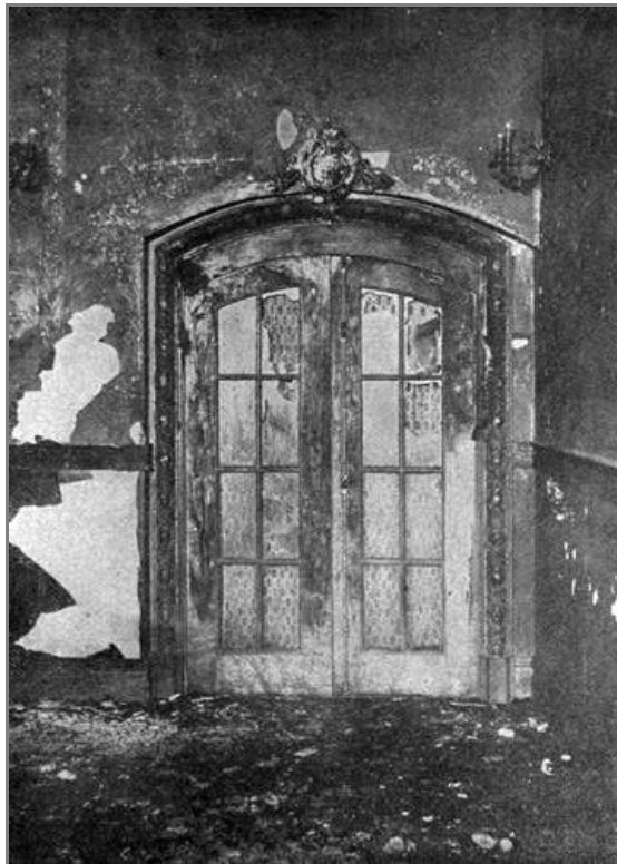
DOOR TO THE FIRE ESCAPE THAT COULD NOT BE OPENED; MANY DIED HERE.
