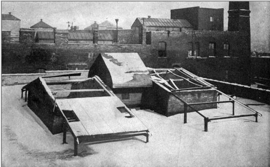
SKYLIGHT ON ROOF OF THEATER, WHICH WAS NAILED DOWN DURING THE FIRE.
