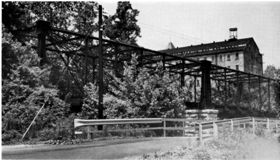
Figure 23.—THE ONLY SURVIVING BOLLMAN TRUSS BRIDGE, at Savage, Maryland. The bridge was built elsewhere in 1852 and was moved to this now-abandoned Baltimore and Ohio industrial siding in about 1888.
