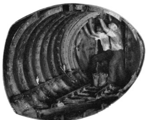
Figure 29.—PLACING A segment of cast-iron lining in Greatehead's Tower Subway, 1869. To the rear is the shield's diaphragm or bulkhead. MHT model—1 ½" scale. (Smithsonian photo 49260-B.)
