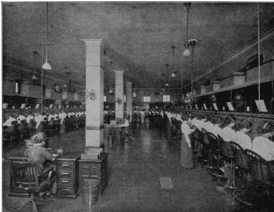
A TYPICAL OPERATING ROOM IN AN AMERICAN CITY, WITH THE MOST MODERN BELL SWITCHBOARD
