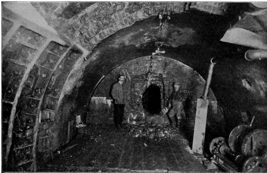
HOLE BROKEN THROUGH THE SOUTH TUBE OF THE NEW YORK AND JERSEY TUNNEL LOOKING WEST
