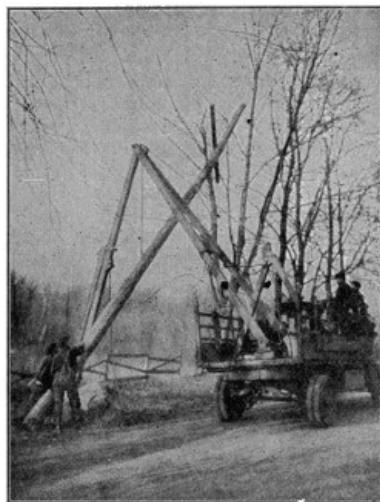
AMERICAN METHOD OF RAISING POLES BY DERRICK WITH POWER FURNISHED BY MOTOR-TRUCK.
