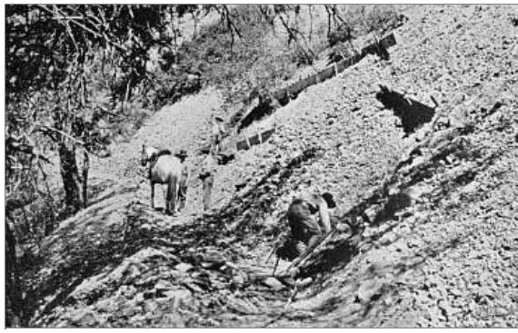
Figure 18. Forest officers and laborers building a wagon road through trap rock. Payette National Forest, Idaho.
