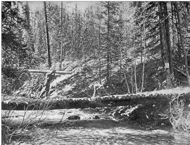
Figure 16. Forest Rangers repairing a bridge over a mountain stream. Arapaho National Forest, Colorado
