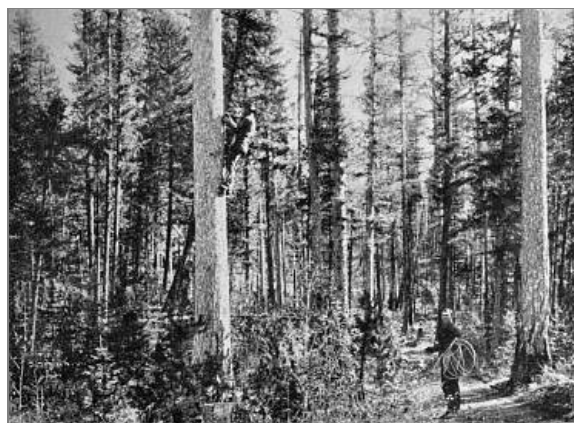
Figure 66. Scene in Montana. Forest officers constructing a telephone line through the Flathead National Forest.
