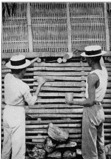
BAMBOO HOUSE SUPPORTS SEALED WITH CEMENT TO PREVENT ENTRANCE OF RATS (MANILA PLAGUE CAMPAIGN)
