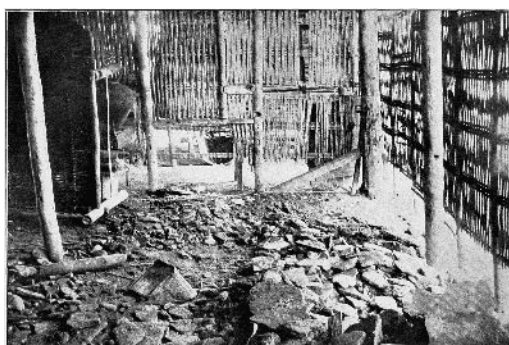
CLEANING AND RAT PROOFING IN BASEMENT OF 1226 CALLE JUAN LUNA IN WHICH TWO CASES OF PLAGUE OCCURRED. RAT CADAVERS FOUND UNDER BROKEN FLOORS (MANILA PLAGUE CAMPAIGN)
