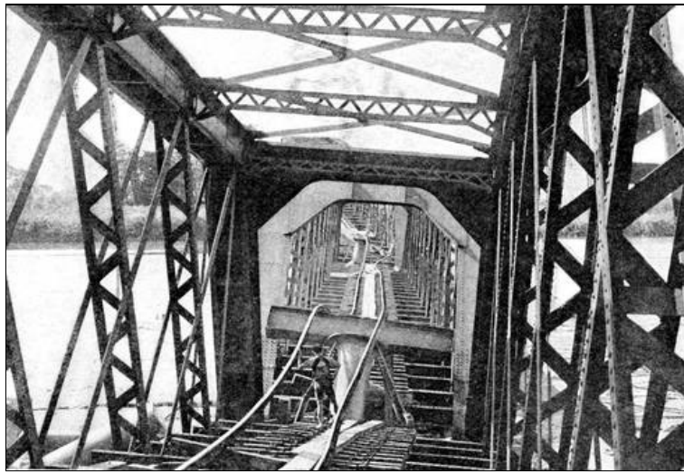
Effect of the Great Earthquake of 1891 on the Nagara Gawa Railway Bridge, Japan.
