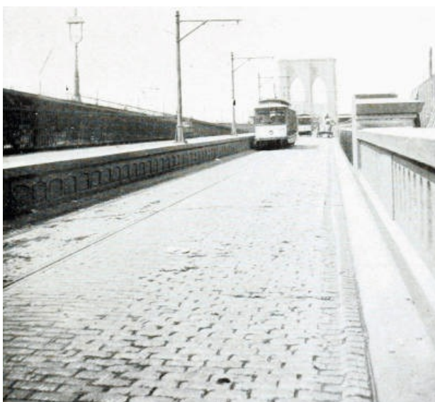
GRANITE PAVEMENT ON ROADWAY OF BROOKLYN BRIDGE AFTER CONSTANT USE WITH VERY HEAVY TRAFFIC FOR SIXTEEN YEARS.
