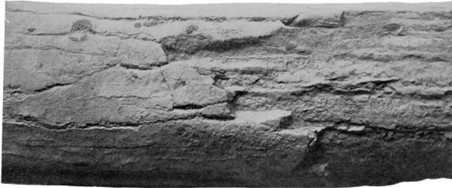
LEAD SERVICE PIPE SHOWING THE DEPTH TO WHICH THE PIPE HAS BEEN AFFECTED.
