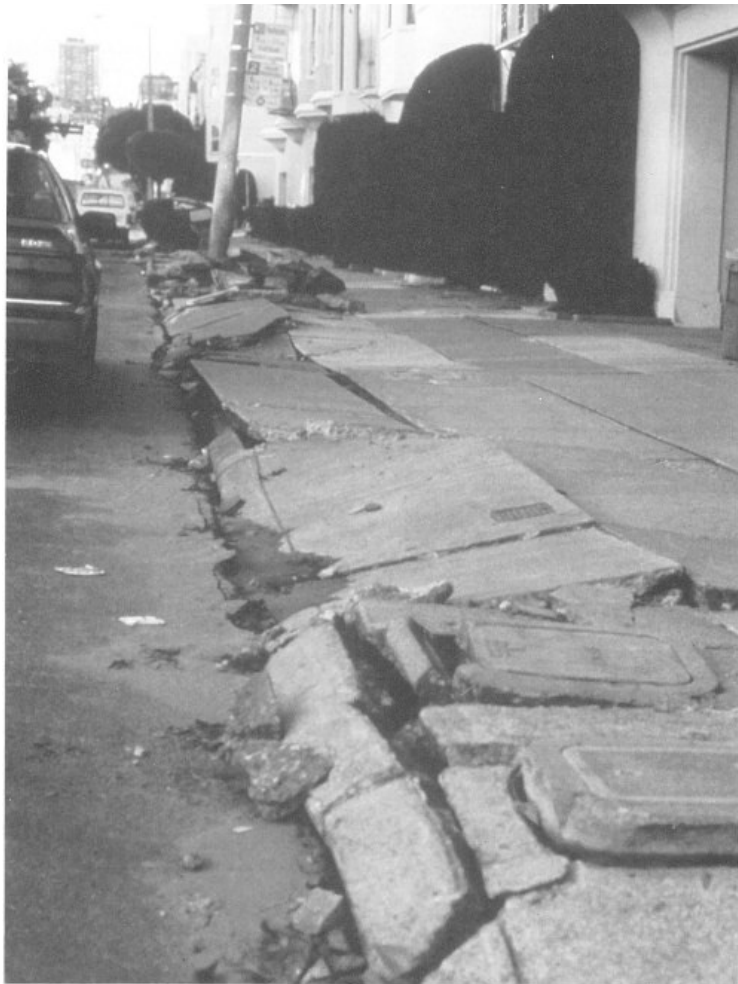
Liquefaction of sands and debris caused major damage throughout the Marina district in San Francisco during the Loma Prieta earthquake.
