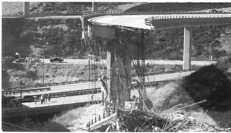
The January 17, 1994, earthquake at Northridge, California, caused this collapse of a major highway interchange. (Photograph by James W. Dewey, USGS.)
