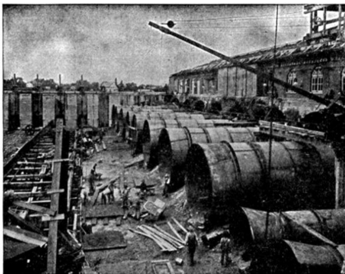
FIG. 36.—Steel Penstocks at Chamblay Power-house.
