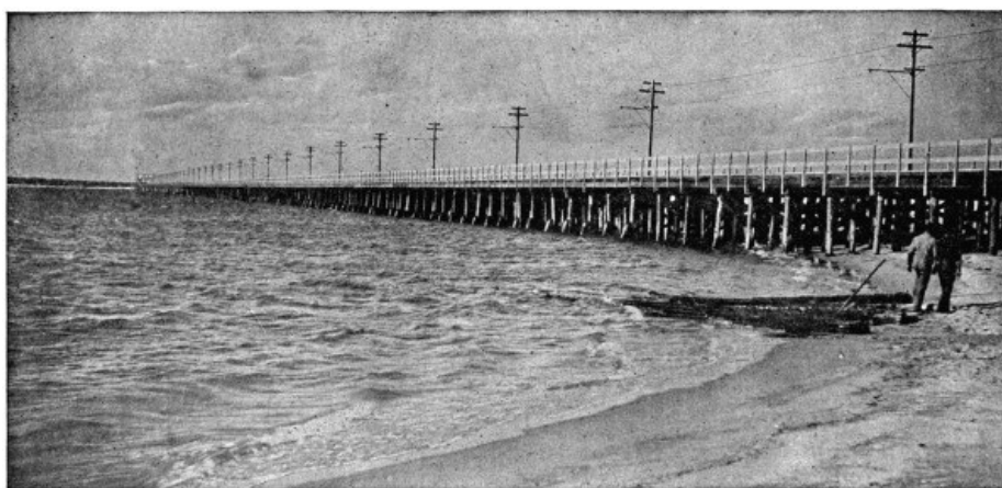
FIG. 80.—Transmission Line of New Hampshire Traction Company over Hampton River Bridge, 4,623 Feet Long.
