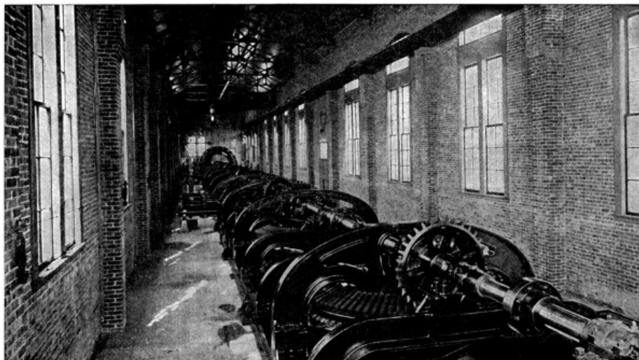
FIG. 30.—Interior of Power-house, Buchanan, Mich.
