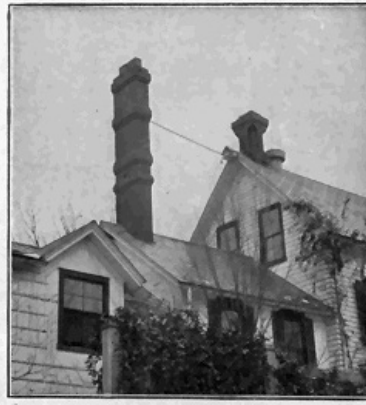
FIGURE 6.—Several extensions were necessary before this chimney would draw properly on account of the wind deflected from the nearby wall.
