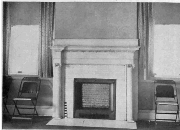
FIGURE 33.—In regions where natural gas is plentiful and in cities, fireplaces of this type, burning gas with a flickering flame, are frequently used as an auxiliary to the main heating plant. Some types have imitation logs of metal perforated for gas jets.
