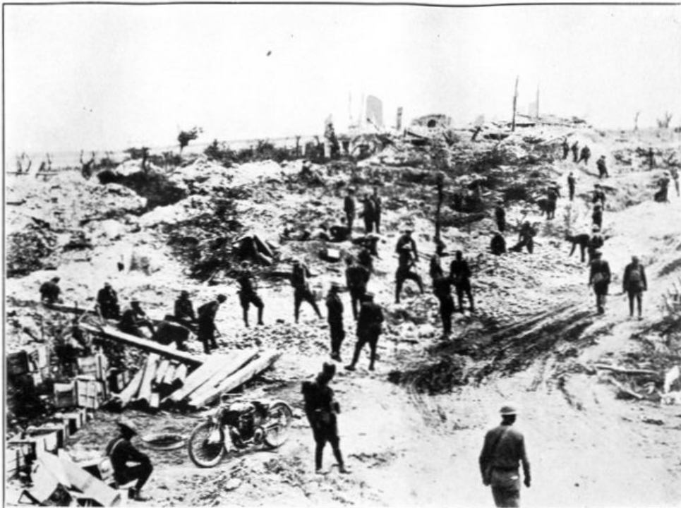
ENGINEERS, ASSISTED BY INFANTRY, BUILDING A ROAD OVER WHAT WAS NO MAN'S LAND ONE WEEK BEFORE.
