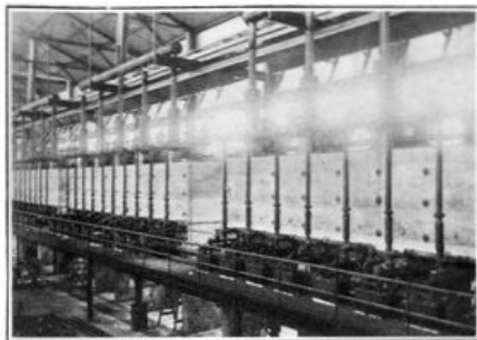
Carbon plant No. 3, showing treater room and west side batteries of Dorsite treaters.
