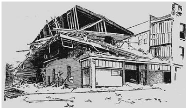
FIG. 86.—Building wrecked at San Mateo, California, during the late earthquake. The heavy roof and upper floor, acting as a unit, have battered down the upper walls (after J. C. Branner).
