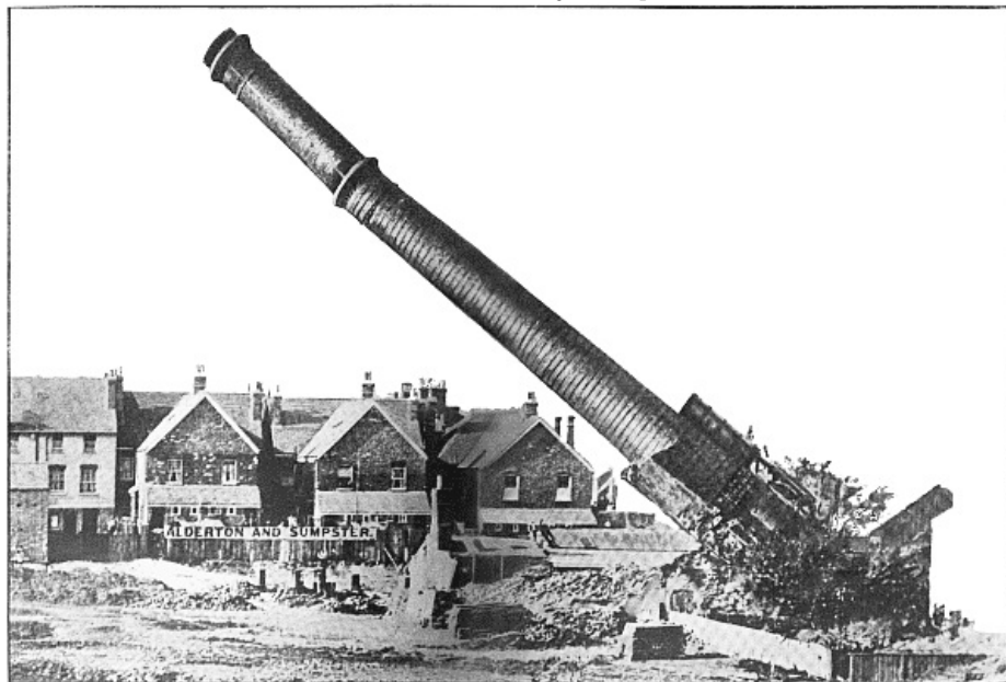
ONE OF THE ALDERSHOT CHIMNEYS FALLING, WATCHED BY AN IMMENSE CROWD—THIS STACK AND ANOTHER FELL EXACTLY UPON THE LINES MARKED OUT FOR THEM.
