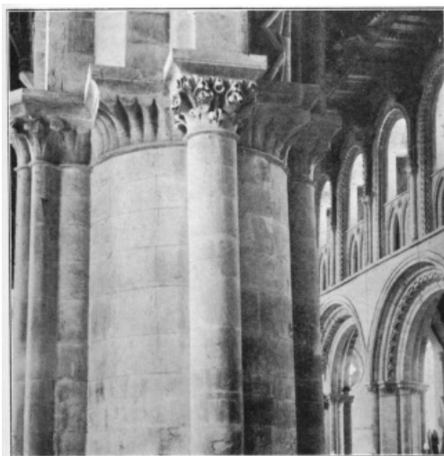
NORMAN SHAFT WITH RE-CARVED CAPITAL, EASTERN PIER IN S. NAVE ARCADE. (See p. 27.)
