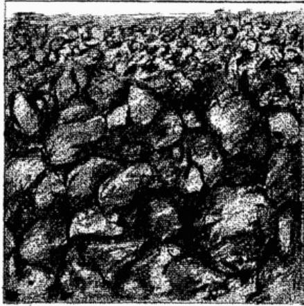
94. To illustrate poor preparation of ground.
